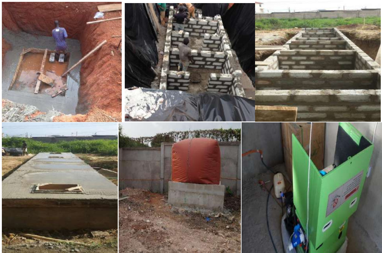
Fig. 5: Construction of septic tank type biogas plant for St. John’s School with balloon & 5KVA generator (counterpart funding)
